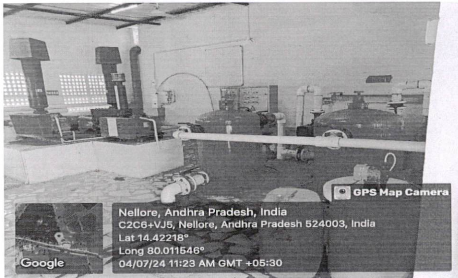
Geotagged photo of inside of sewage treatment plant
